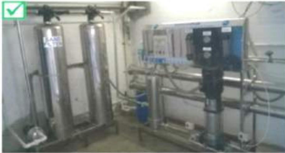
Fig 4.5.5 RO plant for water treatment to meet potable water requirements side the process
